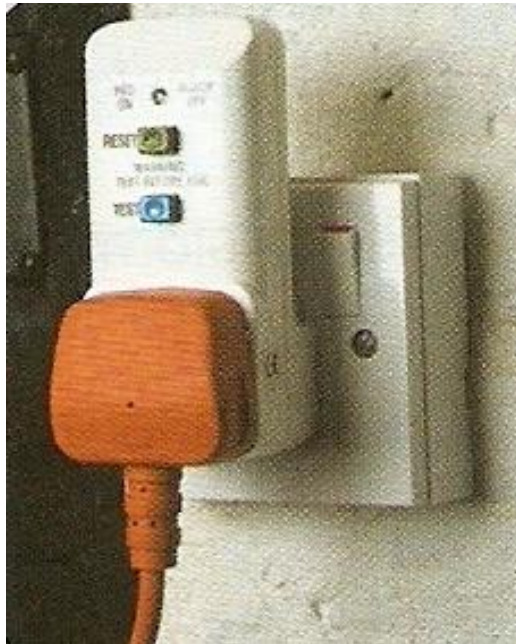
RCD (Residual Current Device) circuit breaker used with an individual appliance
