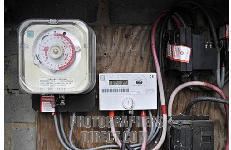
How electricity arrives into our homes
